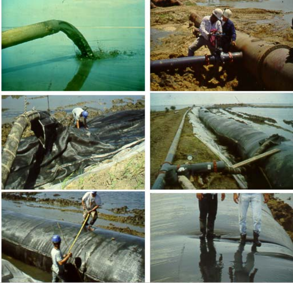
Figure 1b: Clayey Slurry Filled Tubes, Gaillard Island, Mobile, Alabama: Upper Left: Consistency of Dredged Slurry, Upper Right: 8-inch Division Pipe to Supply Slurry to Tube, Middle Left: Flexible Pipe Attached to Inlet Before Pumping of Slurry, Middle Right: Clayey Slurry Pumped through Single Inlet for 2 Hours to Form 150 m Long, 1.5 m High, and 3.6 m Wide Tube, Lower Left: Appearance of Tube Immediately After Completion of Pumping, and Lower Right: Tube Acts as a Filter Allowing Clear Water to Seep Out While Retaining Clayey Particles
