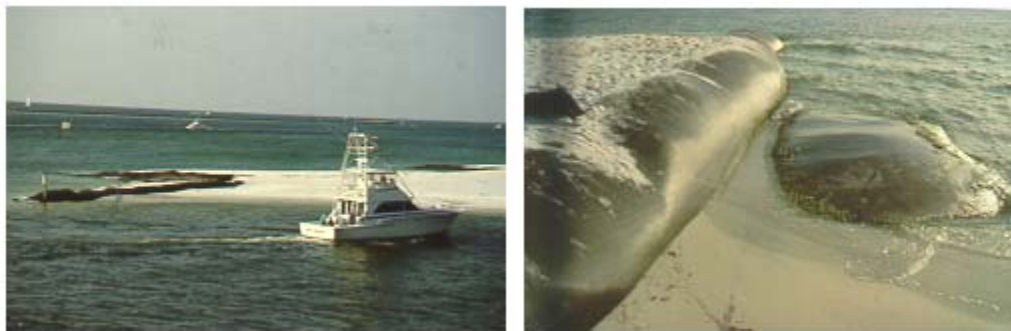
Figure 1a: Sand-Filled Tubes (Groins) to Control Erosion, Destine, Florida: Left: Distant View, and Right: Close-up View
