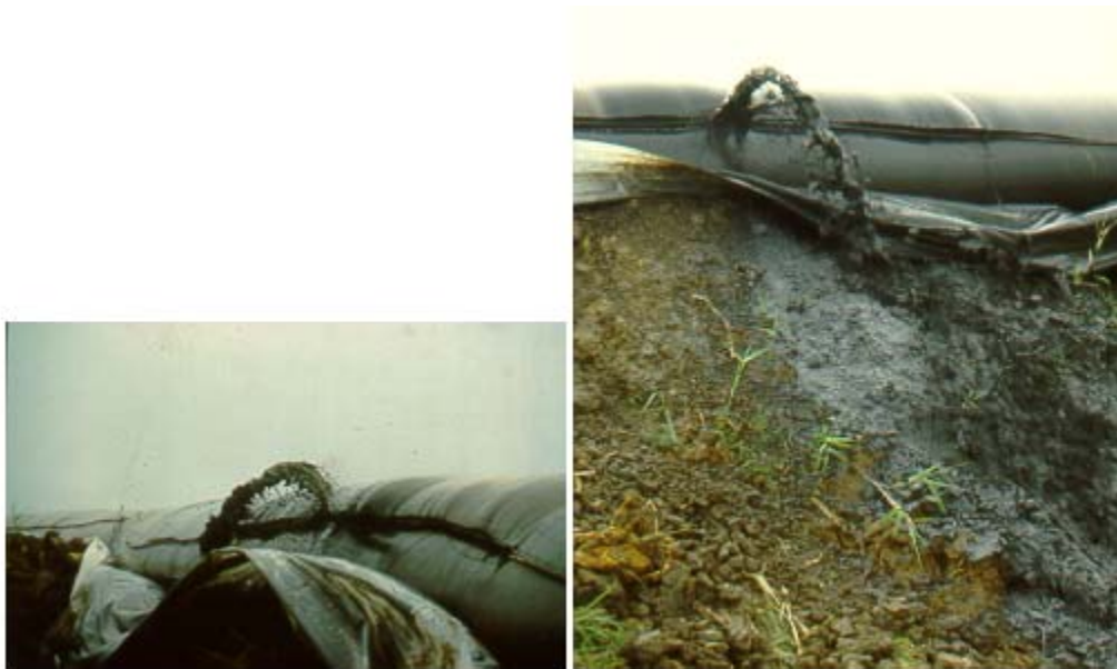
Figure 14. Local Rupture of Defective Seam Due to Slurry Pressure, Gaillard Island, Mobile, Alabama
